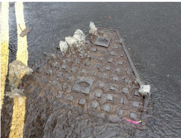
Picture 27 Overflowing storm drain in Ham Ln after moderate rain October 2013
